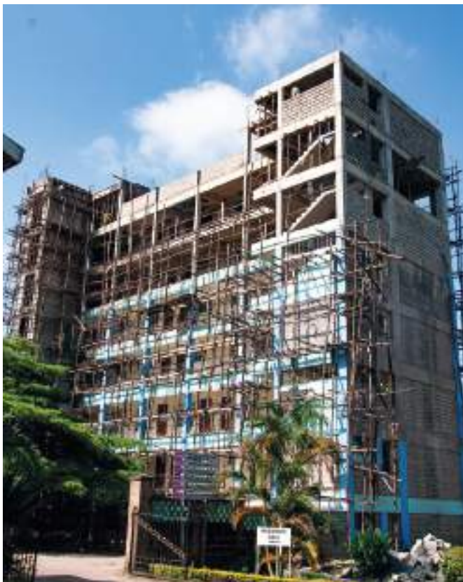
The Camisassa home project under construction at the Consolata Fathers - Regional House in Westlands
