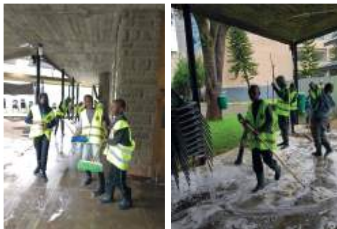
The CMA and Beacon Boys undertook cleaning and unclogging of drainage at the Consolata Shrine.
